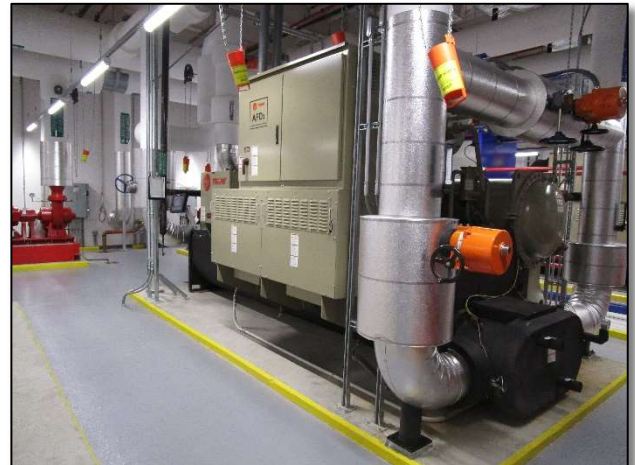
Cloud and colocation data centers are aggressively reducing water usage in new data center designs.
