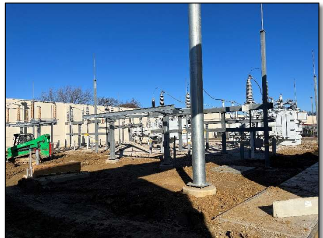
Transformer delivery bottlenecks are delaying new substation energizations and data center expansions
