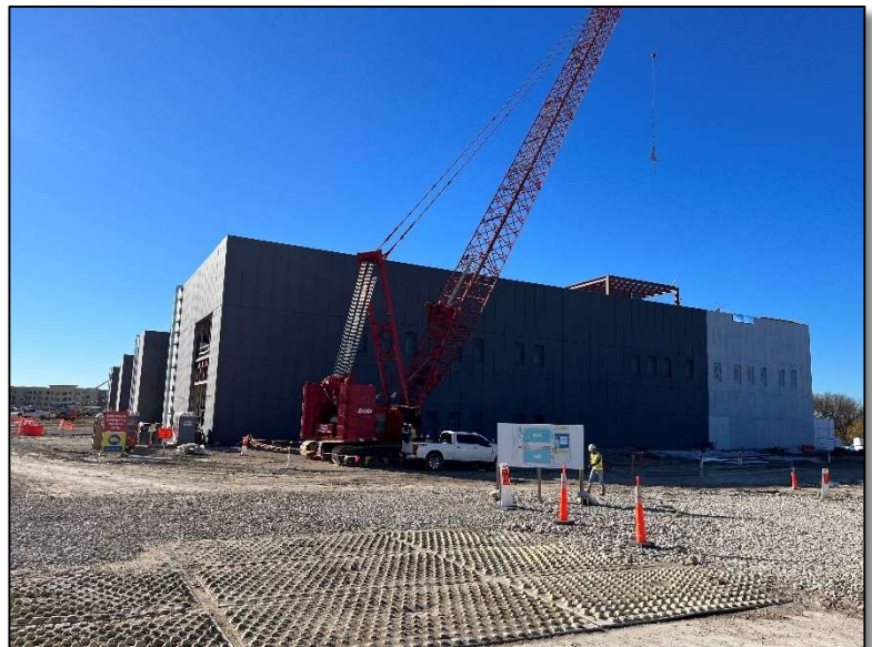
Construction of new data centers is booming worldwide as hyperscale and AI users fuel new facility demand.
